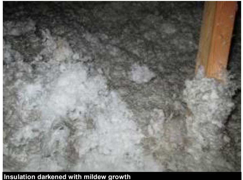
Insulation darkened with mildew growth
