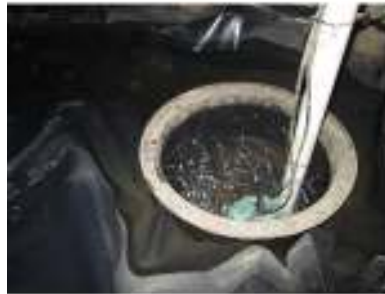
Sump pump and standing water
