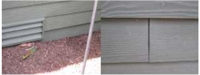
Siding low/Open gaps at siding butt joints
