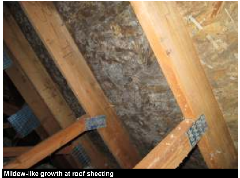
Mildew-like growth at roof sheeting
