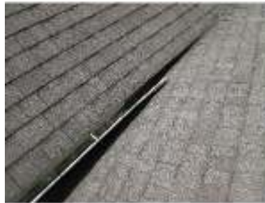
Gutter s blcoked by debris
