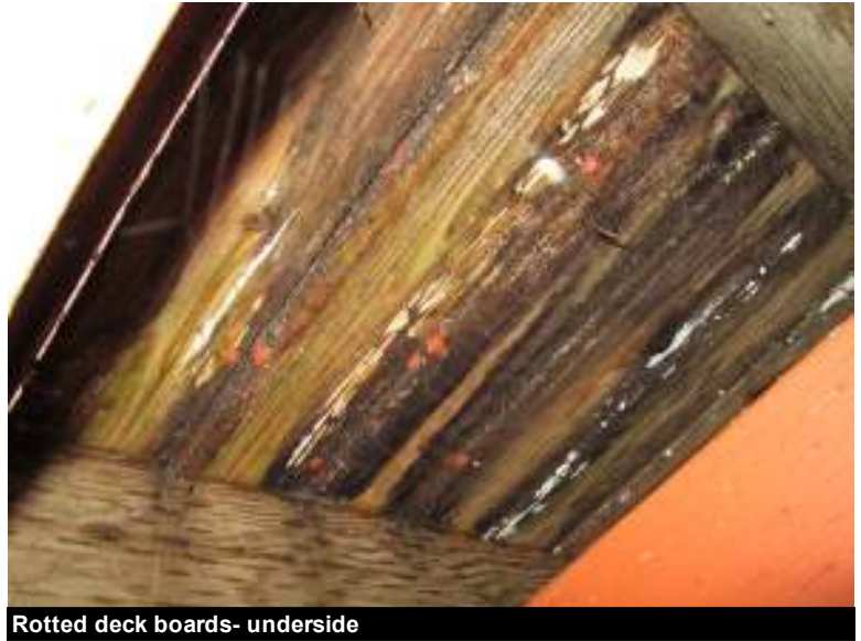
Rotted deck boards- underside
