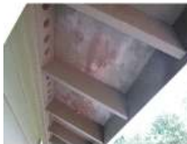
Rotted/wet fascia boards
