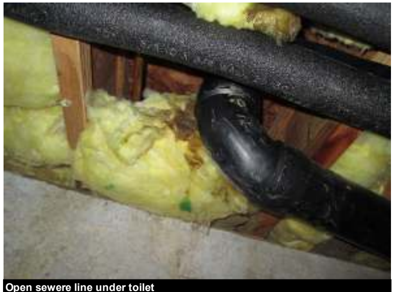
Open sewere line under toilet
