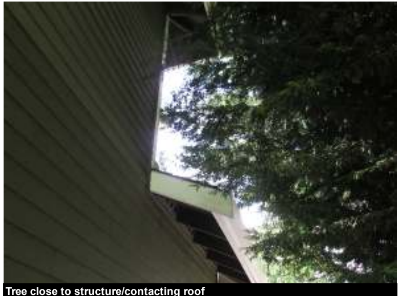
Tree close to structure/contacting roof
